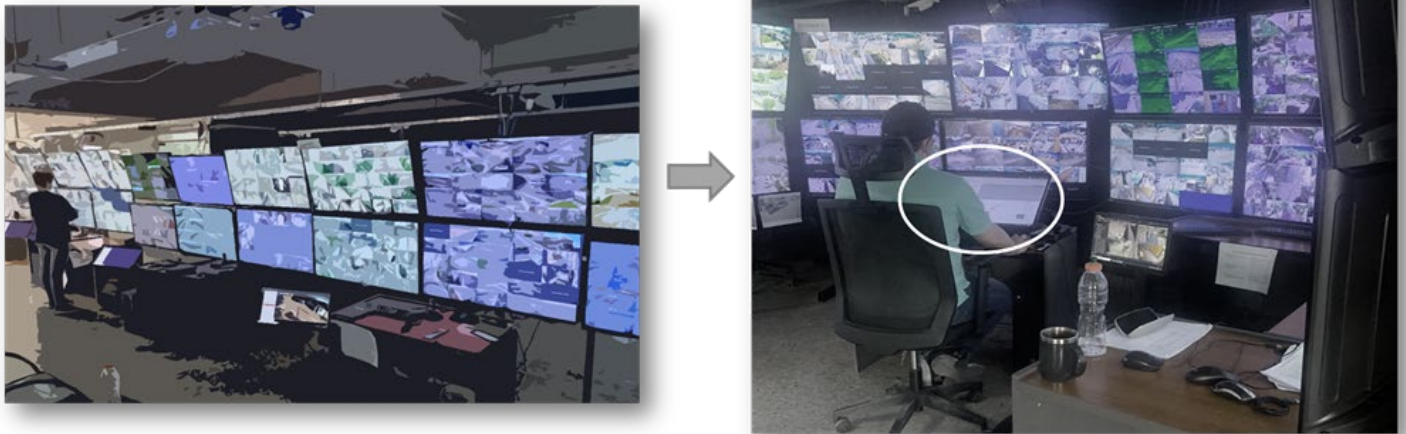
Figure 2. Monitoring Station: An operator utilizing VSaaS alert systems to manage approximately 350 cameras.
