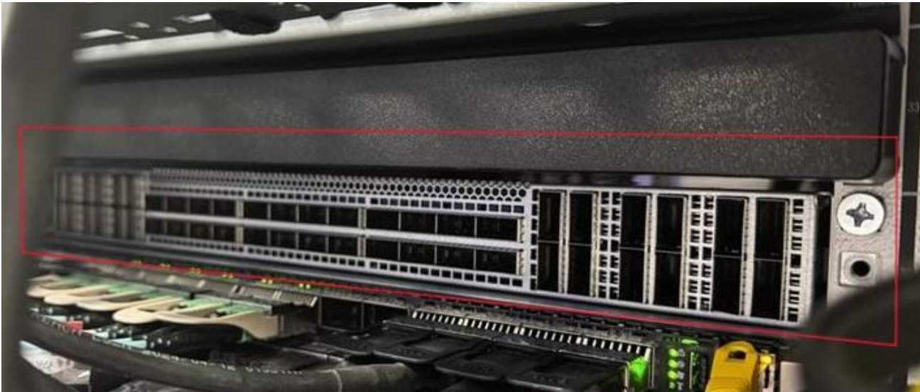
Figure 2 CN5000 Edge switch racked in the Lenovo Benchmarking Centre
