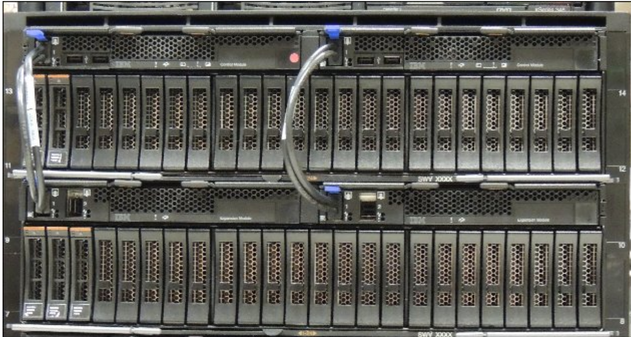
Figure 3. Flex System V7000 control and expansion enclosures
